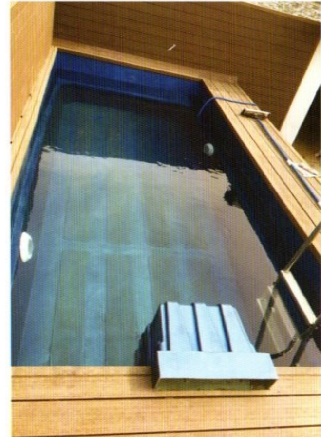
5. Filling the swimming pool and cover it to protect the water from Heat, Cold and Dust.
