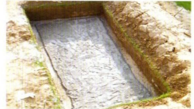
3. Preparation of Ground after excavation with PCC/RCC on the floor before placing the swimming pool.
